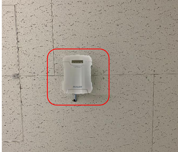
View looking up at receiver installation location from the shop floor.
